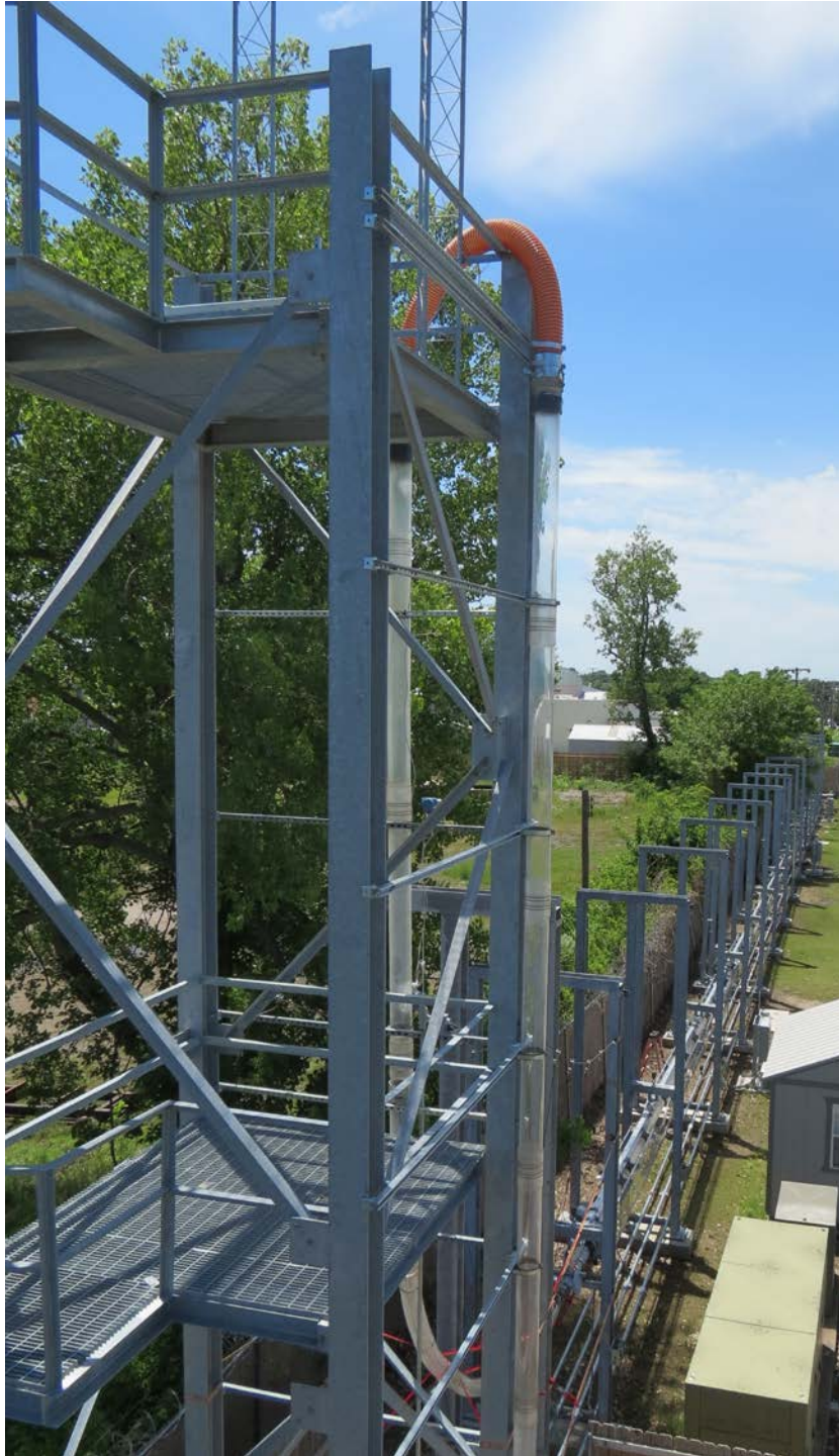
Figure 6. View of 6-in. Horizontal Well Facility
